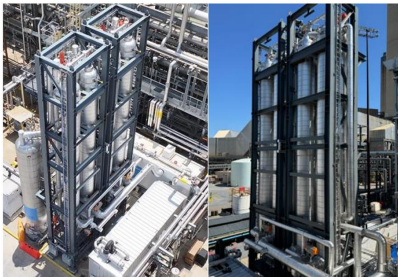
Figure 2 FrostCC™ Pilot Plant Installed at the National Carbon Capture Center
