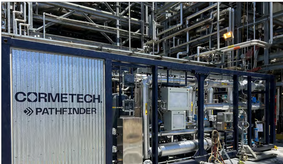
Figure 15. Installed CORMETECH Skid
