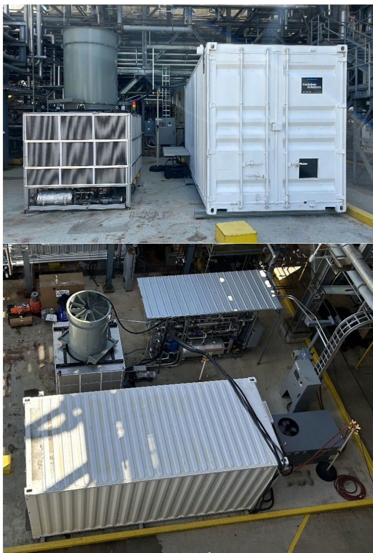
Figure 13 – DAC-100, Heat Skid, and Liquefaction container installed and operational at the NCCC
