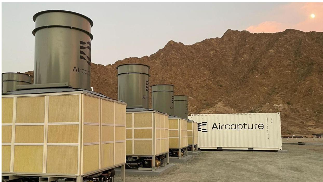
Figure 17 – Project Hajar during commissioning in October 2024
