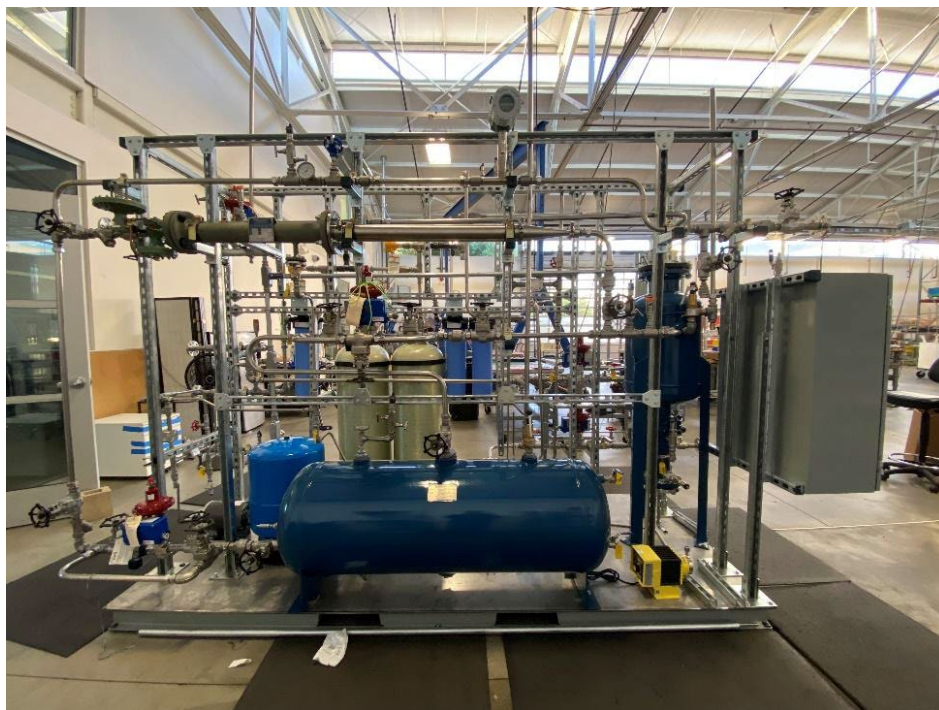
Figure 8 – Completed Heat Integration Skid
