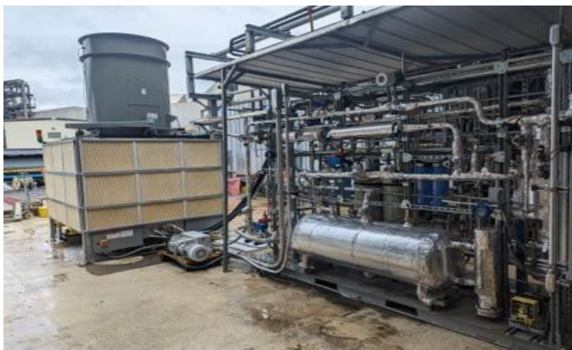
Figure 12 – DAC-100 and Heat Skid installed and operational at the NCCC
